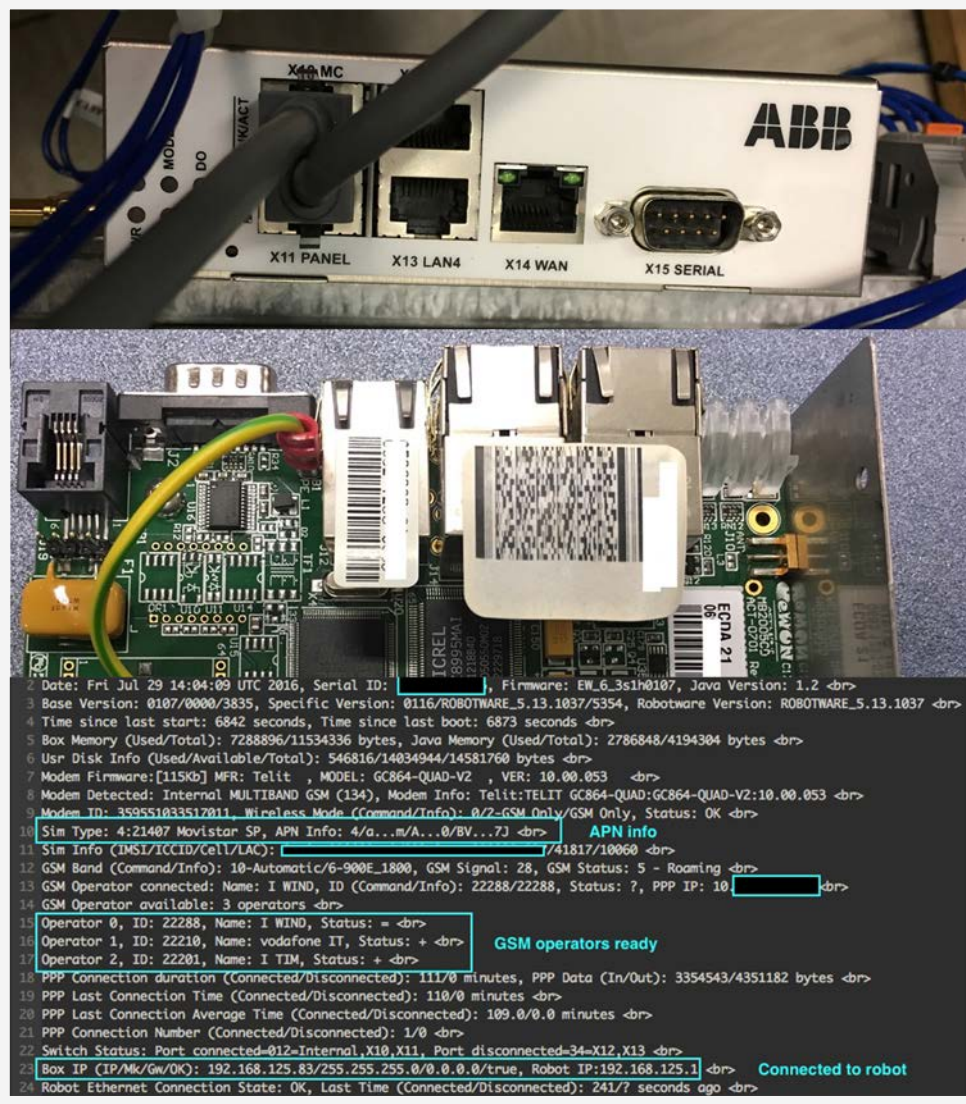
Figure 16. ABB's Service Box (a rebranded eWON industrial cellular router) attached to our robot with system logs that show the connection to the robot via the service APN
